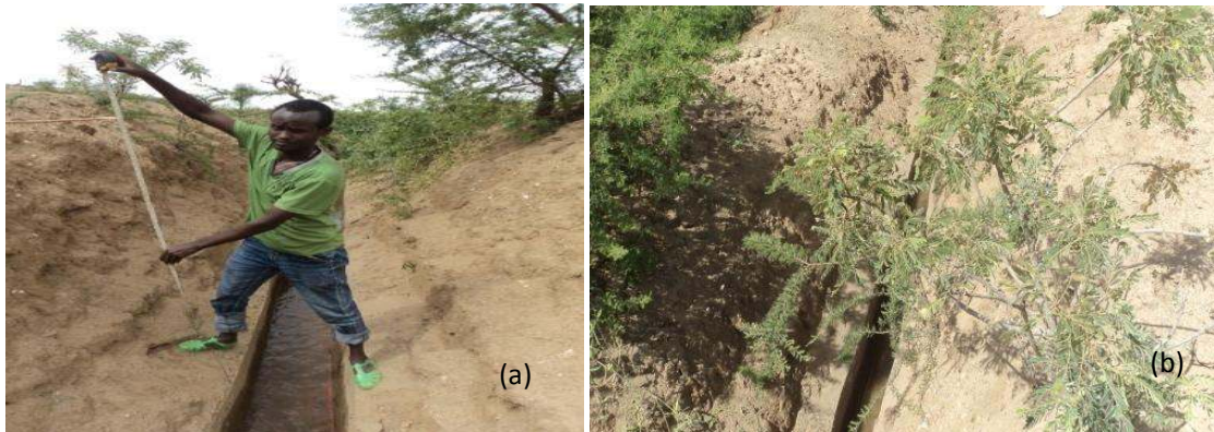
Fig. 4. The main cause of the mal-functionality due to depth of irrigation canal below OGL
