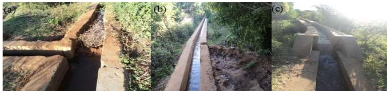
Figure 4. Main causes of hydraulic structure mal-functioning of T.Tsalit SSI scheme.
