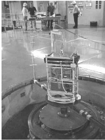
Fig. 10. Measurement Control unit.
