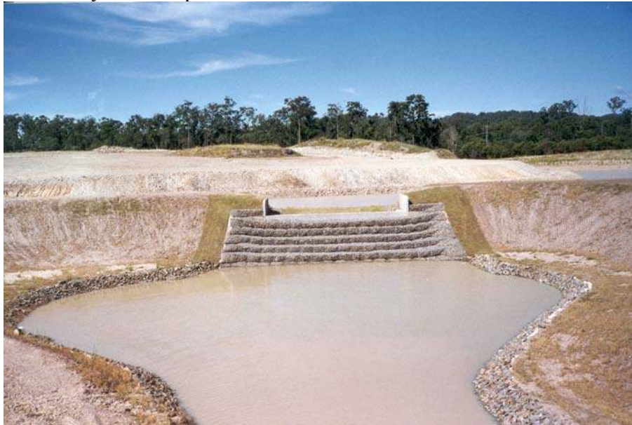
Fig. 1 - Gabion stepped weir at Robina, Gold Coast (Australia) - h = 0.6 m, l = 1.1 to 2 m (A) On 2 April 1997 shortly after completion
