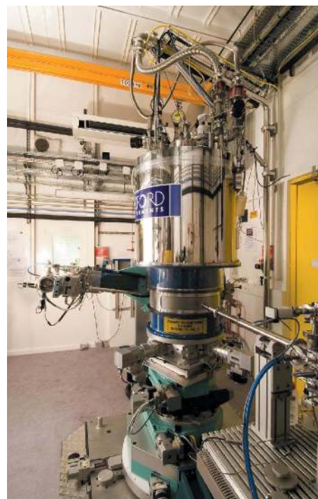
Figure 9 The 10 T split-coil superconducting magnet installed in EH2. All the magnet services including leads, vacuum tubes, gases and electrical connections come from the top and are connected by a pivoting vacuum arm fixed on the wall.
