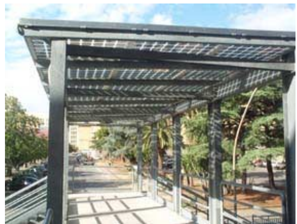
Fig. 1. View of the PV array.
