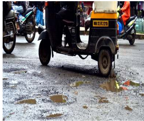
Fig. 3. Potholes and damaged roads
