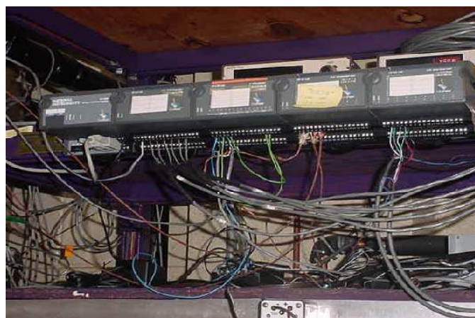
Figure 15: Field Point Data Acquisition Hardware (H)
