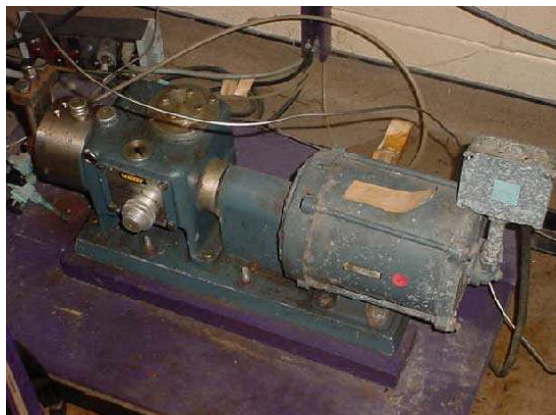
Figure 13: Cleanup Centrifugal Pump (F)
