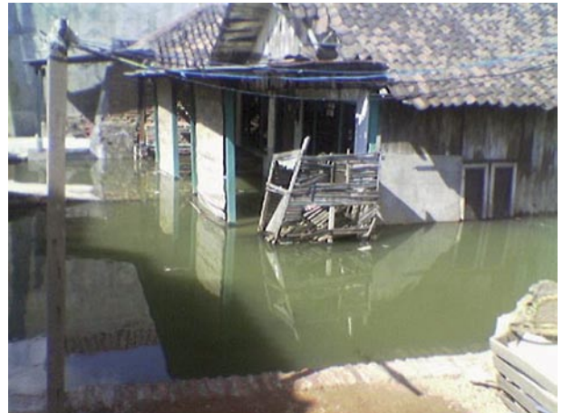
Fig. 10. House damage due to tidal inundation.
