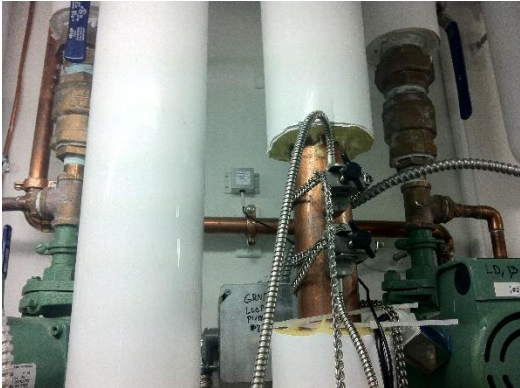
Figure 11 Transducer unit 4 on the wall of mechanical room
