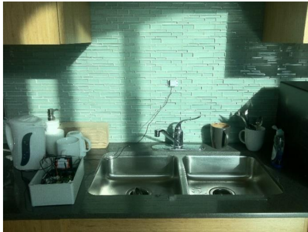
Figure 7 Transducer unit 8 on the wall of kitchen room
