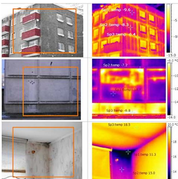
Fig. 4. Thermal bridges of a concrete element apartment building from outside (top and middle) and from inside (bottom)
