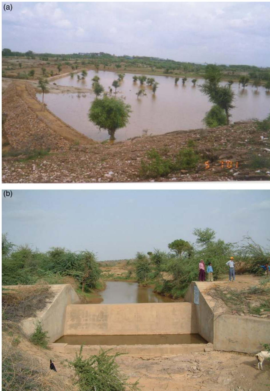
Figure 2. The village tank constructed for harvesting runoff using (a) masonry and earthen embankments and (b) check dam on a stream.
