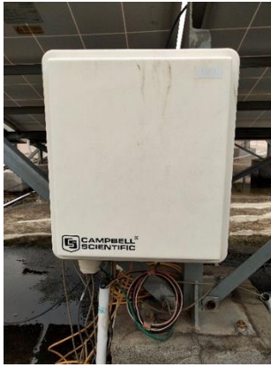
Figure 6. CR3000 data logger
