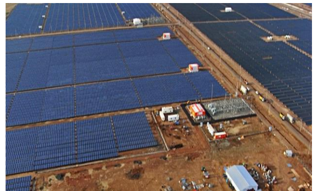
Fig. 1 Aerial View of 5 MW Gujarat Power Cooperation Limited Solar Photovoltaic Power Plant
