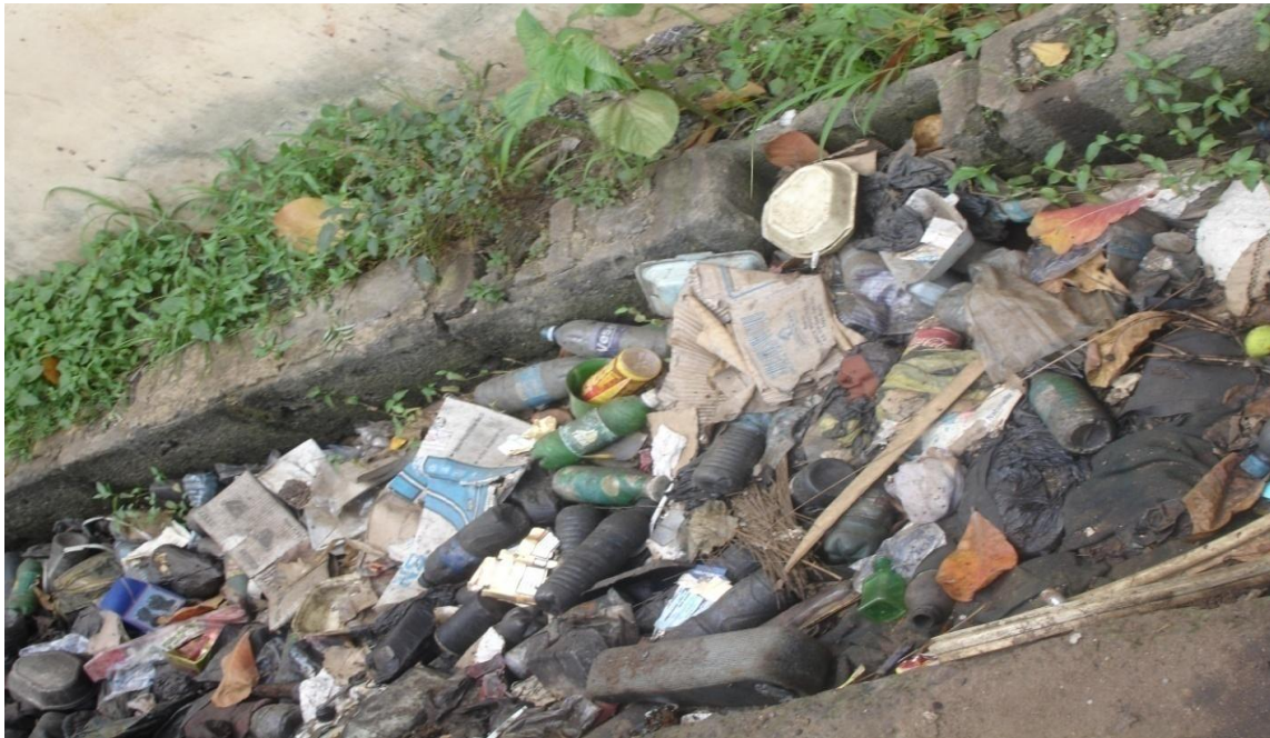
Plate 1. Blocked Drainage System in Agege
