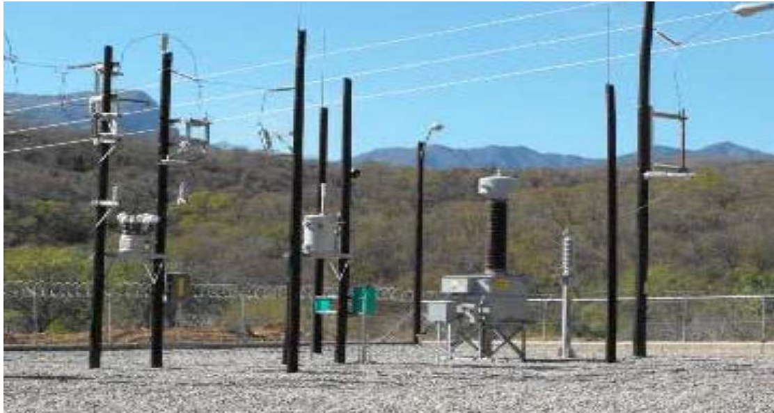
Figure 2. Auxiliary service voltage transformer (ASVT)
