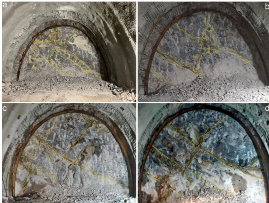
Fig. 13 Injection dispersions encountered during tunnel excavation (a-Km:54 + 049,00, b-Km: 54 + 028.25, c-Km: 54 + 004.25, d-Km:53 + 990.75 excavation face, injection are the areas within the yellow lines)
