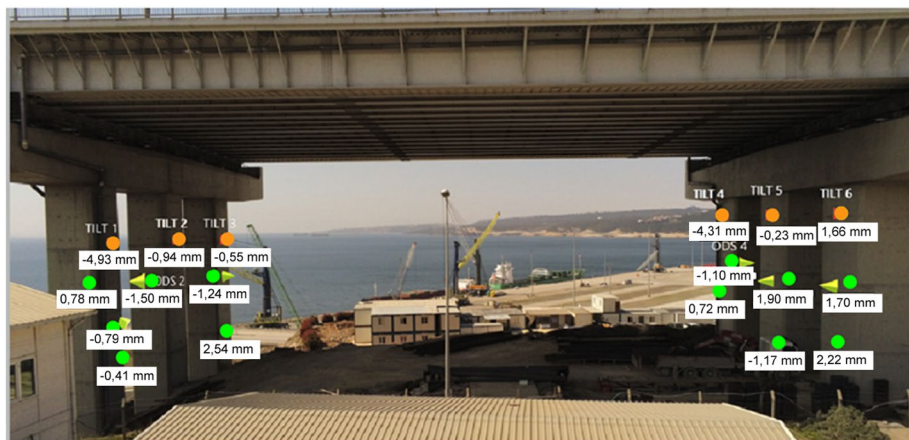
Fig. 17 Readings dated (01.06.2022) after the completion of the tunnel from tiltmeters and ODSs placed on Viaduct P-02 and P-03 legs (Orange dots show Tilt Meters, green dots show ODS points, yellow arrows show the direction of movement)
