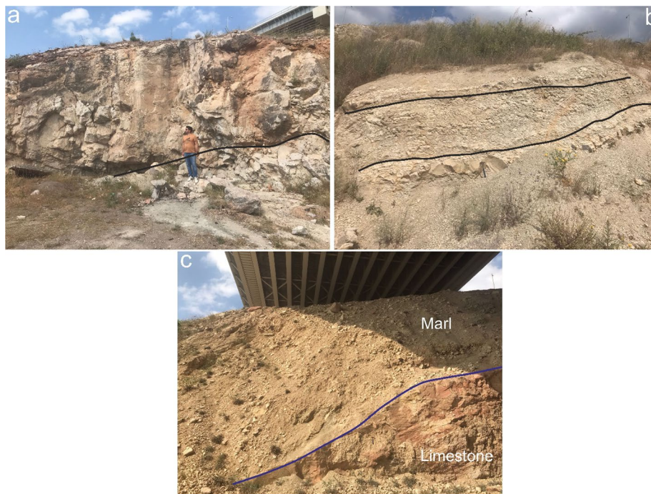
Fig. 3 Geological units observed around the tunnel (a: dolomitic limestone, b: marl, c: boundary between limestone and marl, black line: layers, blue line: shear zone)
