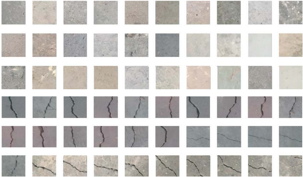
FIGURE 3: Crack image sample.
