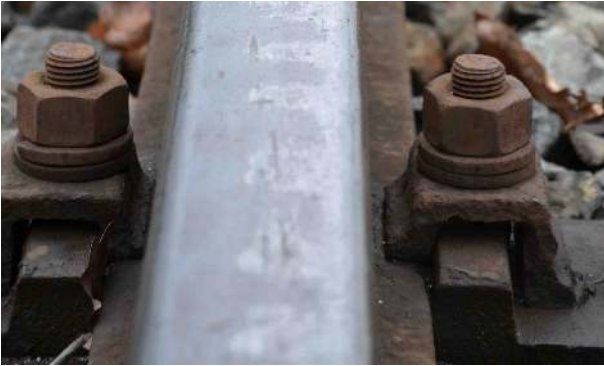
Figure 1. Corrugated rails reduce the driving comfort in terms of vibration and noise while increasing the overall wear due to harsher track - train interactions.
