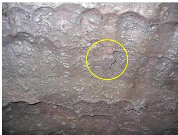
Figure 2. Slagging gasifier refractory sidewall showing corrosive wear and spalling (circled material).
