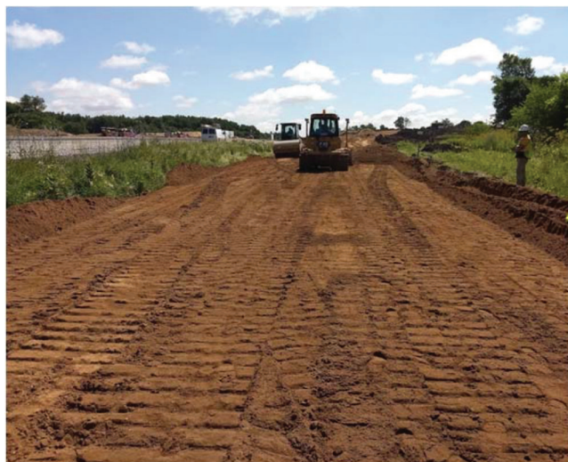
Figure 7.5 Subgrade compaction for No. 30 backfill soil using vibratory compactor for the construction of a ramp at US 20 and IN 2 intersection at Rolling Prairie, IN.
