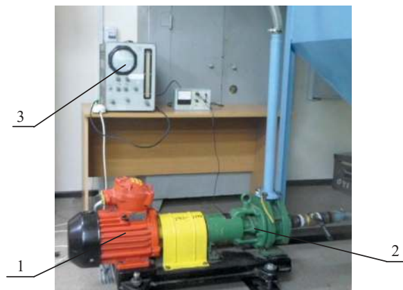
Fig. 11. Installation measuring system: 1 – electric motor, 2 – pump, 3 – vibrometer
