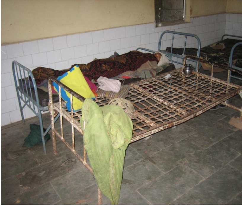
XIV. CHC Garhokota, district Sagar, Madhya Pradesh, February 2009 - Maternity ward beds without mattresses and no doctor available at the CHC, which is a 24X7 facility.
