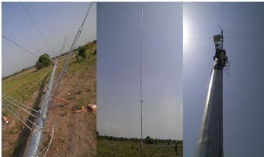
Fig.10. NRG 60 m wind energy masts XHD.
