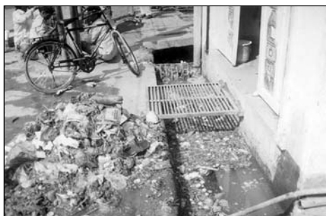
Waste is discharged into drains.
