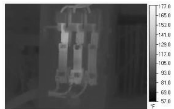
Fig. 3 After cleaning center fuse contact showing decrease of 70 deg. in temperature
