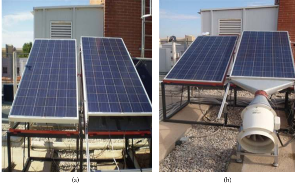
FIGURE 1: Solar experimental facility. Left panel labelled as panel A is not modified and the right panel labelled as panel B is above a steel plate, creating an air channel underneath it. (a) Natural convection configuration. (b) Forced convection configuration.
