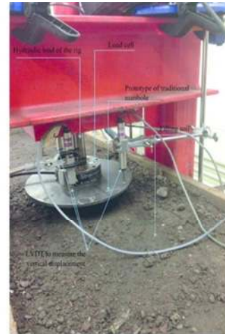
Fig. 7 b. Setup of the trench in the rig and location of measurement instruments on the traditional manhole surface at three points on the edge.
