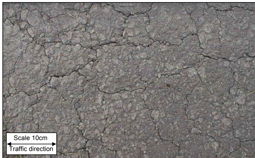
Figure 11. Final crocodile crack pattern observed at 'failure' of road section.
