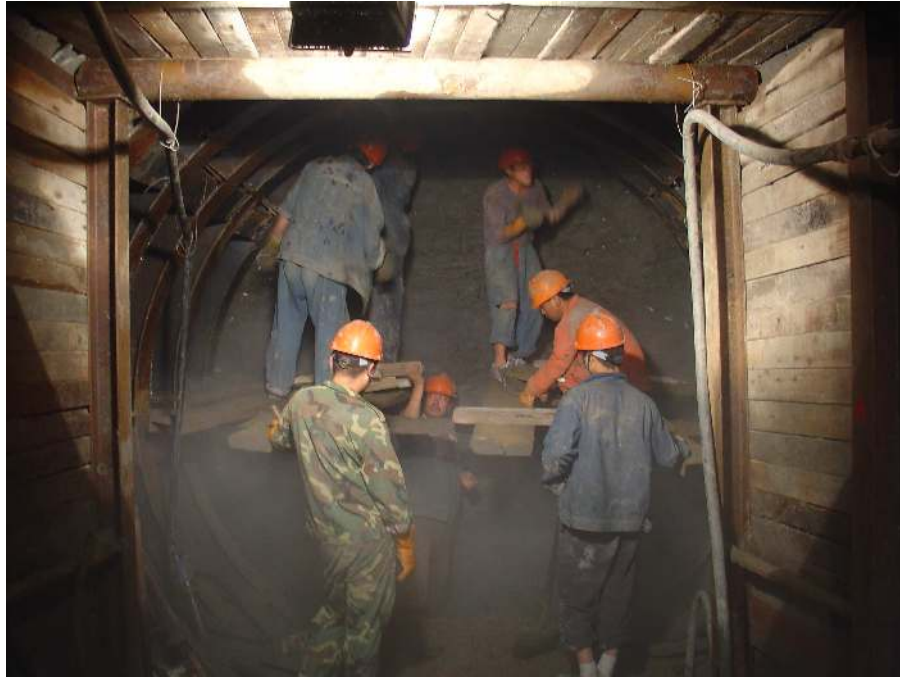
Photo 1. Excavation of cross passage for Shanghai Yangtze River Tunnel by the mining method
