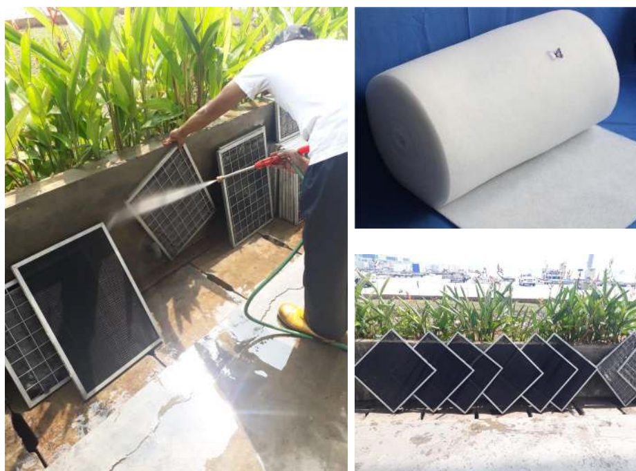
Figure 4. Filters being cleaned at the terminal.
