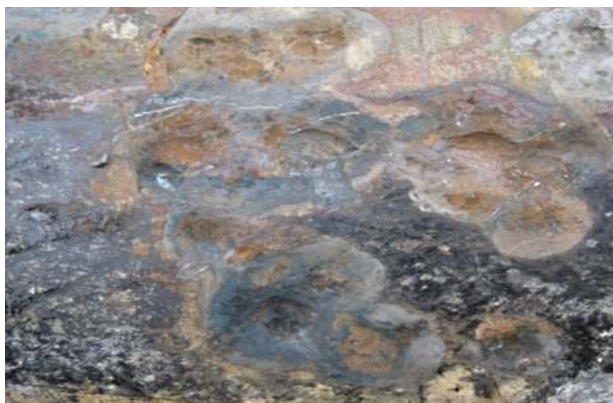
Fig. 1. Corrosion ulcers found on the wall of the gas main "Pasichna – Tysmenytsia"
