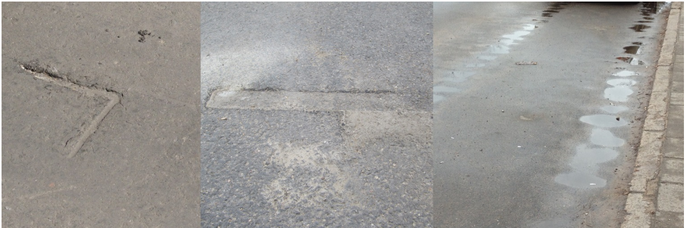
Fig. 2. Permanent deformations of pavement effected by static and impact loading
