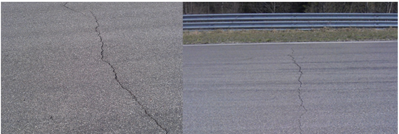
Fig. 3. Thermal cracking of asphalt pavements
