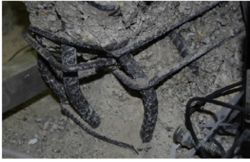
Fig. 1. Damage in slender RC walls due to bar buckling [3]
