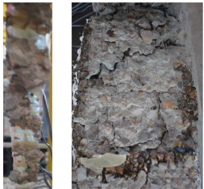
Fig. 12—Failure surfaces after 10,000 hours. Cycles -10 and 30°C (14 and 86°F). Strips 20 and 80 mm (0.787 and 3.150 in.).
