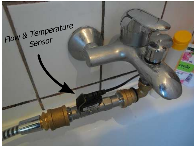
Figure 8: Picture of the installed Resol Grundfos flow sensor in the circuit between tap and shower head.
