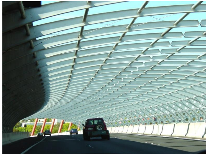
Figure 1.1 Acoustic barriers on the Tullamarine Freeway, Melbourne Australia (Photo; Atlantica). For some burdens such as noise there are engineering solutions available assuming sufficient mitigation costs are included in the initial project appraisal. Others such as the impact of automobile emissions and the particulate matter they produce on air quality may require policy action to limit certain vehicles and to encourage modal shift to less polluting forms of transport.
