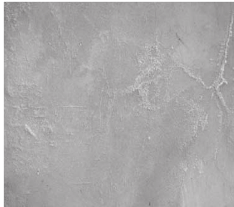
Figure 4: Efflorescences in the rendering cracks.
