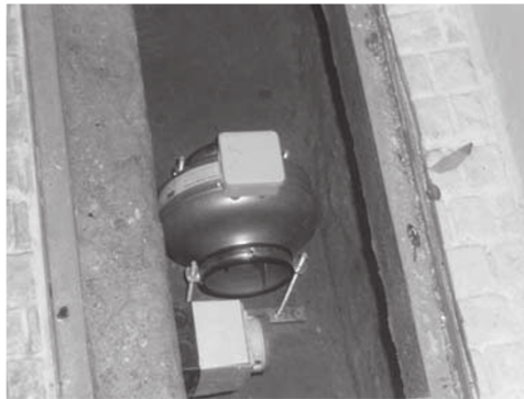
Figure 14: Electric equipment to force ventilation.
