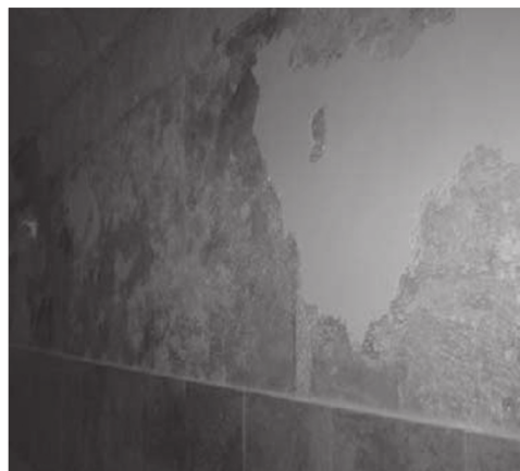
Figure 5: Detachments (large lacuna) of internal finishing.
