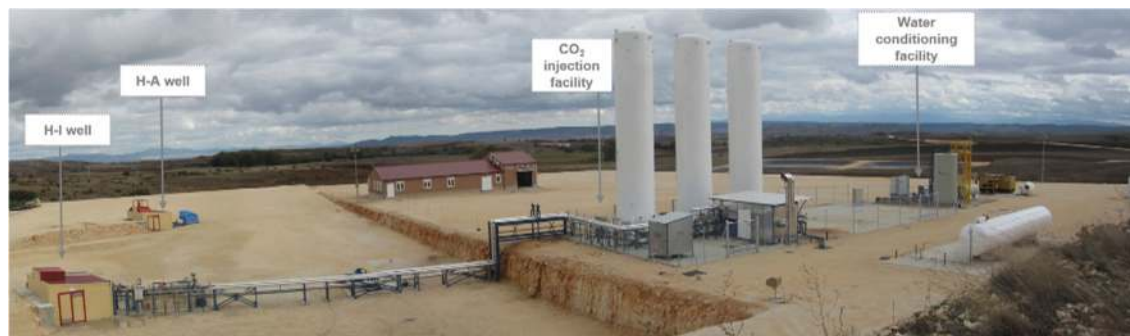
Fig 2.-Schemes of injection well HI (left side) observation well HA (right side) and panoramic view of the pilot
