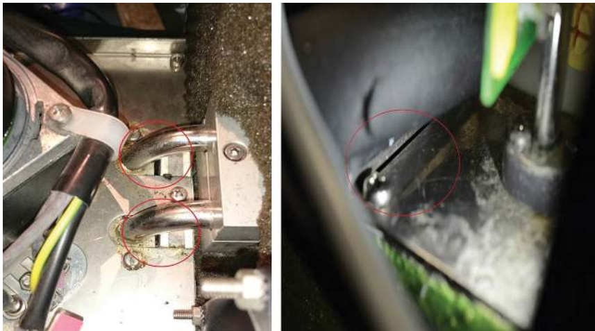
Figure 1. Holes (highlighted by the red circles) close to the flow and return pipes of both heater-cooler circuits and gap between tank sealing plates identified by an aerodynamic particle sizer as areas of aerosol release.
