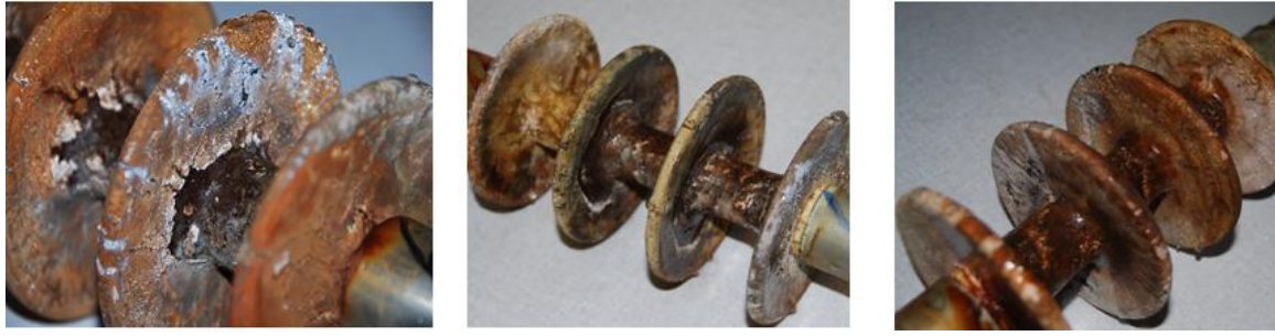
Figure 5.30: Comparison of hydrophobicity for the RTV SR coated porcelain insulator (channel 6) with a unified SCD of 28 mm/kV for HVAC and positive and negative polarity HVDC excitation
