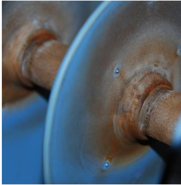
Figure 4.33: Detailed view of aging of the HTV SR insulator (Channel 4) for HVAC excitation
