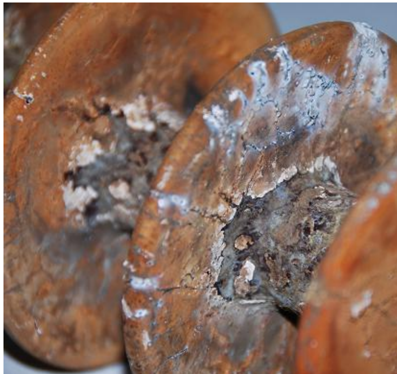
Figure 4.38: Detailed view of aging of the RTV SR coated porcelain (Channel 6) insulator for HVAC excitation
