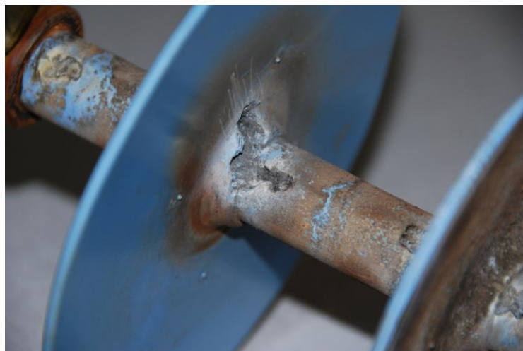
Figure 4.22: The puncture on Channel 3 (HTV SR insulator with SCD of 28 mm/kV) for HVAC excitation
