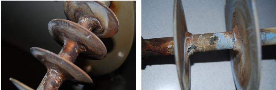
Figure 4.78: Channel 2 and Channel 3 after the test with negative polarity HVDC excitation
