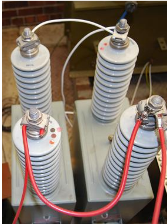
Figure 3.7: The smoothing capacitor bank
