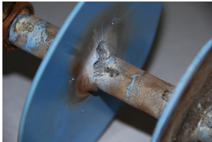
Figure 4.30: Detailed view of aging of the HTV SR insulator (Channel 3) for HVAC excitation
