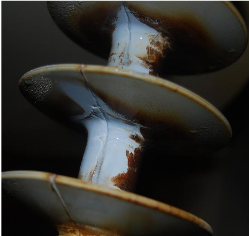
Figure 4.72: Detailed view of aging of the EPDM insulator (Channel 1) for negative polarity HVDC excitation
