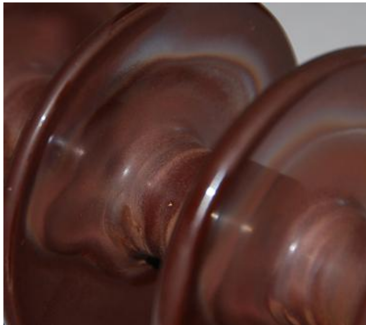
Figure 4.36: Detailed view of aging of the reference porcelain insulator (Channel 5) for HVAC excitation
