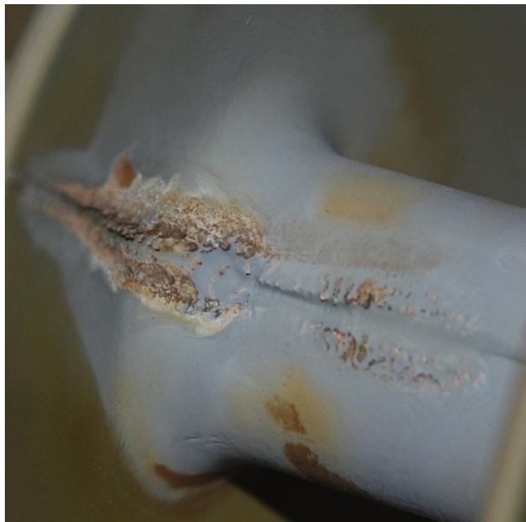
Figure 4.25: Detailed view of aging of the EPDM insulator (Channel 1) for HVAC excitation
