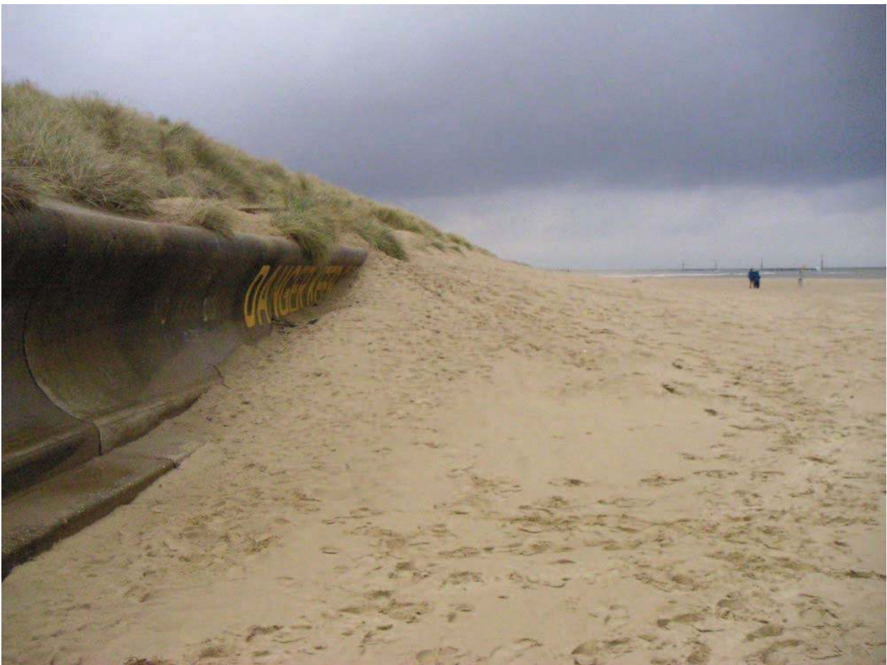
Figure 2 Beach at Winterton with concrete sea wall in front of sand dune on 31 st October 2003 (the detached breakwaters are just visible on the horizon)
