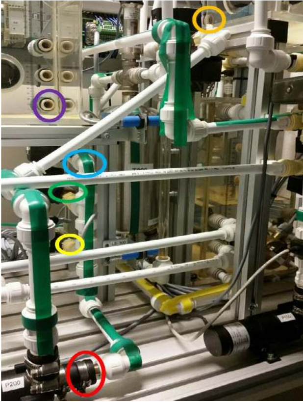
Fig. 11. Marking the color coded nodes and edges in Fig. 10 with colored ellipses on the relevant process components on the photo of the pipeline.
