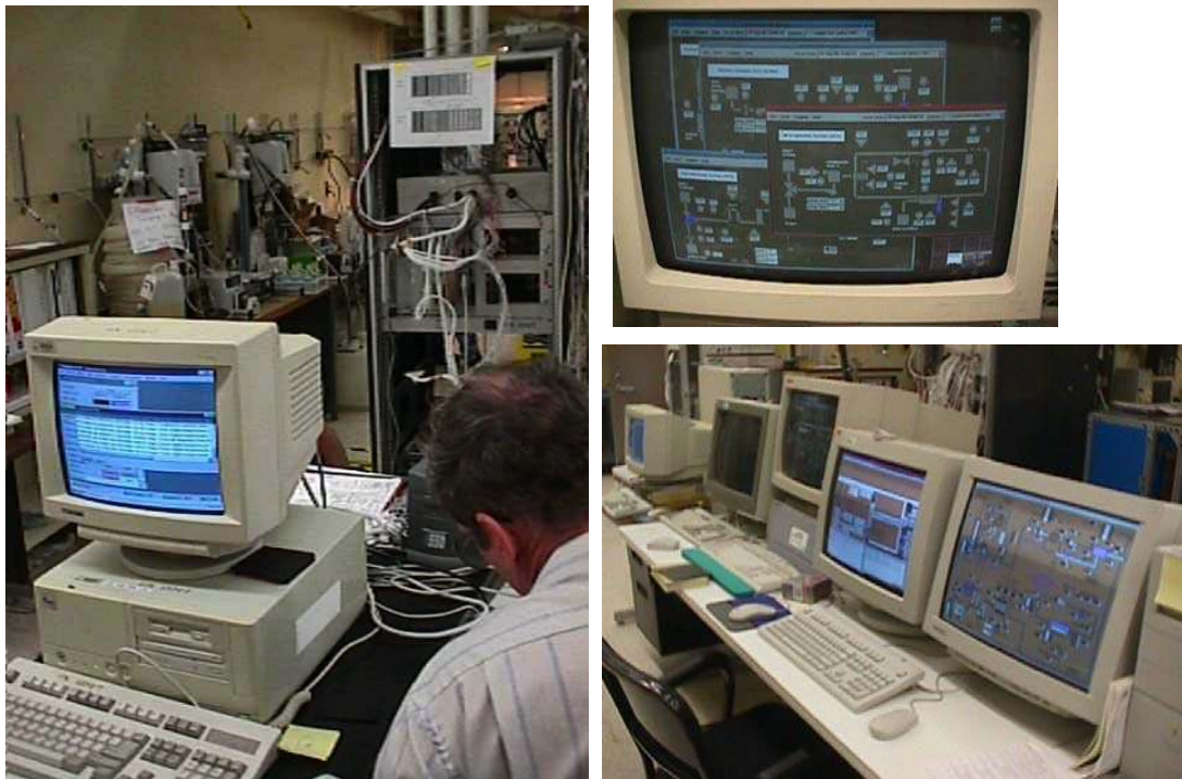
Figure 7 3T Control Computers for the iWRS. On the left is a view of the 3T VME Rack behind the computer that is used as a secondary interface to the RO high-pressure pump. On the right is a view of the (unattended) 3T control table. From foreground to back, the displays are two sequencer/planner displays, the IPC/skill manager display, the display of the broadcast server, and a display associated with the high-pressure pump used in the RO. In the upper right is the display showing the graphical user interfaces (GUIs) for each subsystem generated by the data broadcast from each skill manager.
