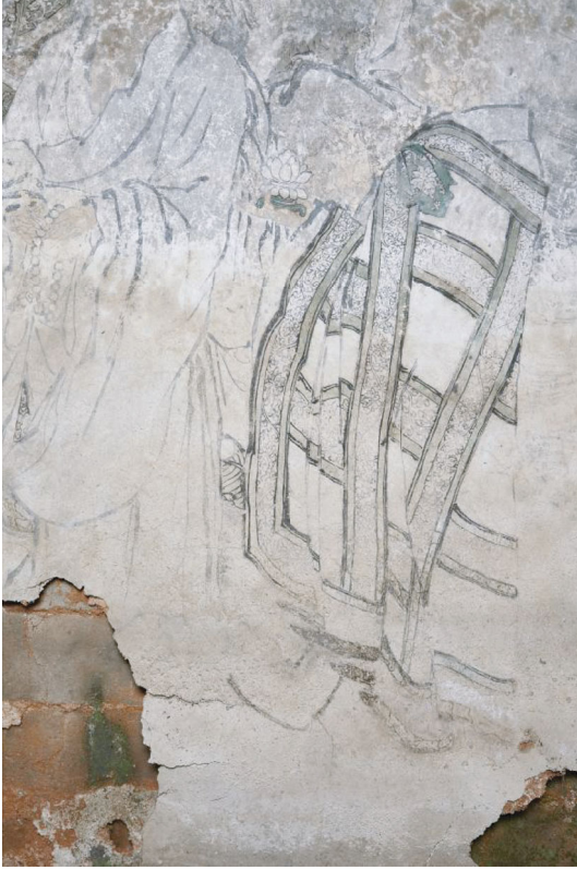
FIGURE 1: Hollowing and falling off of mural image.
