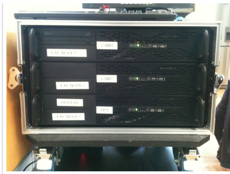
Figure 31 Flumotion Venue Nodes (Rack 1): Three rack machines – two for camera capture and encoding, one for VGA capture and encoding.
