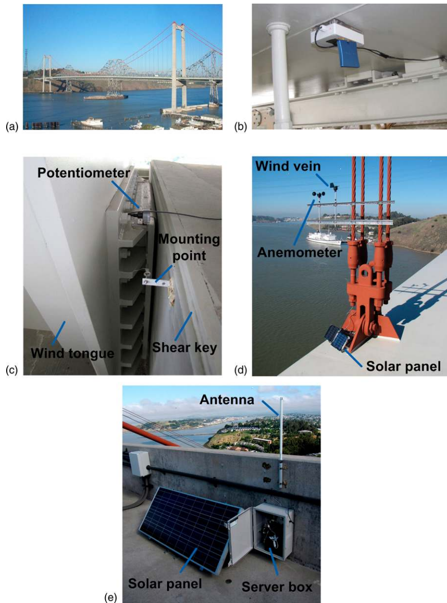
Fig. 3. (a) View of the NCB bridge from Crockett, California; (b) Narada sensor node magnetically mounted to the bottom surface of the main steel orthotropic deck; (c) installation of potentiometer at the north tower shear key; (d) installation of climate sensors (vane and anemometer shown) and solar panel at one of the bridge hangers; (e) Narada server, solar panel, and antenna anchored to the top of the north concrete tower
