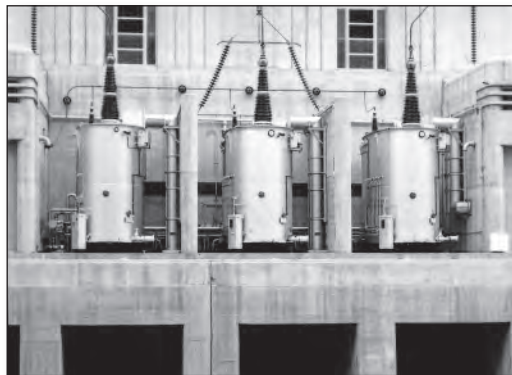
Hoover Dam transformer bank, Units A1 and A2, showing A-phase transformer with the new heat exchange unit installed. Photograph by Bureau of Reclamation.
