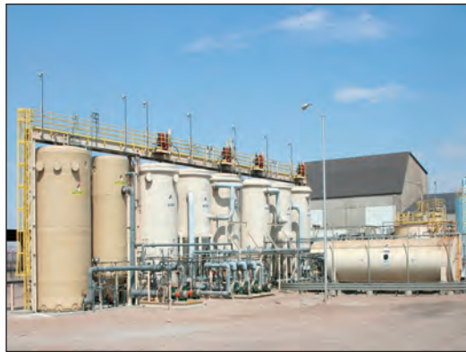
Treatment facility for bioremediation of perchlorate in Henderson, Nevada. Photograph provided by Nevada Division of Environmental Protection, Bureau of Corrective Actions, Special Projects Branch.
