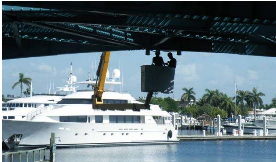
Figure 95. Sensor installation at the movable bridge
