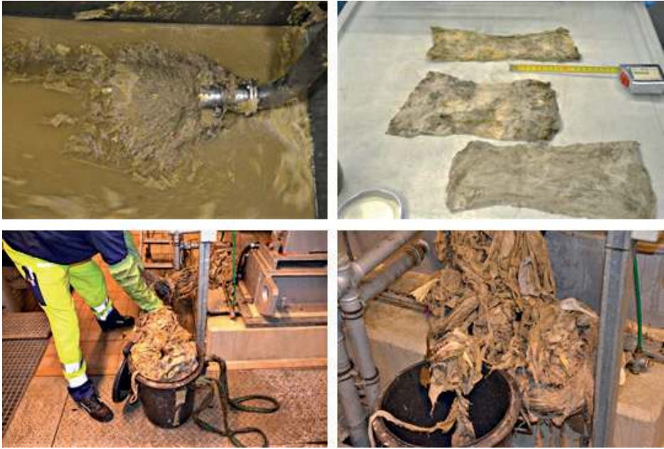
Fig. 4. Impressions of wet wipes in the Berlin sewer system [pictures from TUB-FSD and BWB]
